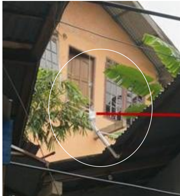
Figure 7: Installed Antenna at Batu Ampar, Batam, Indonesia
