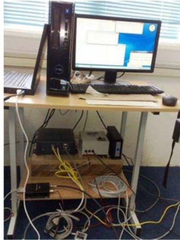
Figure 2 : AIS Installation in the UTM, Marine Technology Center
